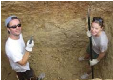
Graham Forman and Amy Hughes digging a latrine for the new high-school in Jinocua.
